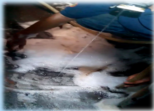
d. Leakage Occurred
